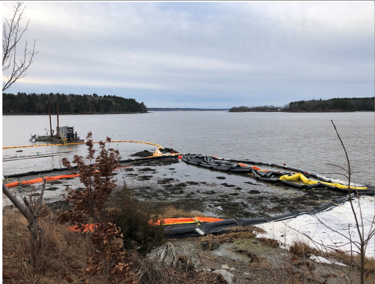
Replacement silt curtain using segments of the turbidity barrier and Type 1 silt curtain. Remainder of the northern segment of the turbidity barrier was secured to the north of the work area.
